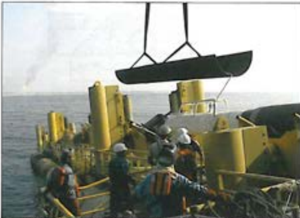
A view of the Startup Head Protector during installation under the Startup Head
