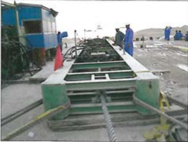
General view of the Linear Winch
