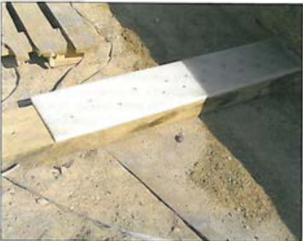
Pipeline extending over wooden traverse on shore
