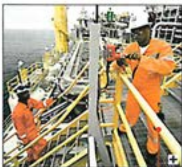
Laurindo Pemba (left) and Guilherme Pascoal perform maintenance aboard the FPSO, center of Kizomba A's production operations
